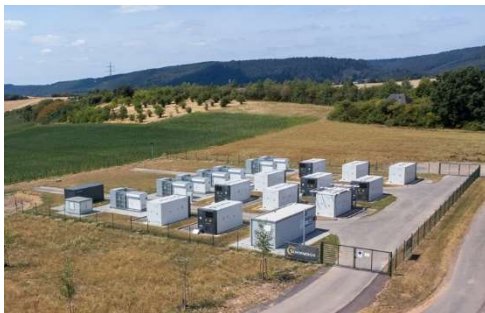
Fig. 2 Large-scale battery storage facilities, such as this one in Föhren, Rhineland-Palatinate, play an important role in ensuring the stability of the power grid. © Fraunhofer ISE
