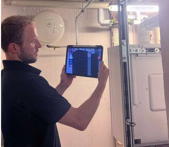
Fig. 1: The “Heat Pump PlanAR” app is being tested in the boiler room. The components of the heating system diagram are projected onto the background using augmented reality. © Fraunhofer ISE/ modified with AI support
