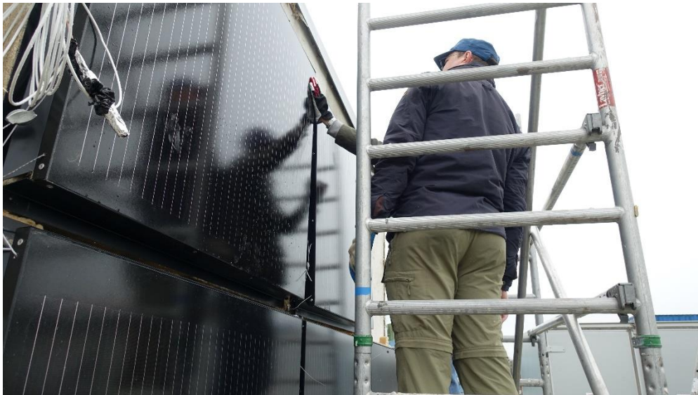
Installation of the PV elements. The research team developed a variant with an insulating material made of hemp fibers and a variant made of mushroom material. © Fraunhofer ISE / Photo: Mona Mühlich
