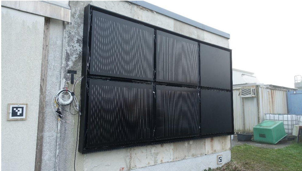
Demonstration installation of six PV façade elements at the Fraunhofer IBP location. The amount of PV elements can be extended as required, colored as needed and installed quickly. © Fraunhofer ISE / Photo: Mona Mühlich
