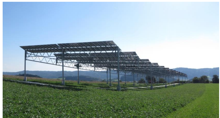
The agrophotovoltaics (APV) pilot plant located in Heggelbach near Lake Constance couples the production of electricity and food crops. ©Fraunhofer ISE
