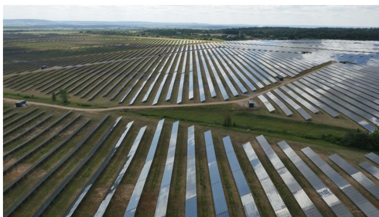
Solar PV power plant in Toul, France (115 MWp) ©EDF Energies Nouvelles
