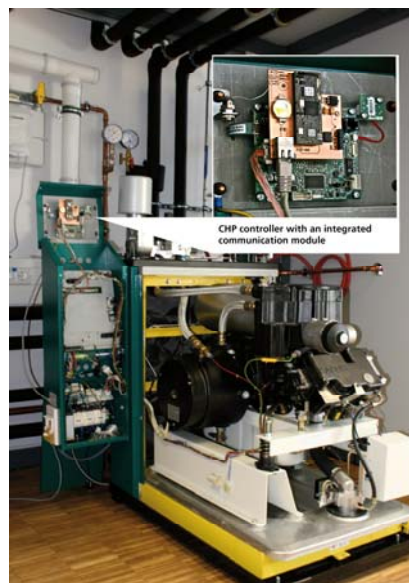
Fig. 2: The project partners developed a controller with a communication module for CHP plants such as this "SenerTec Dachs" unit which is suitable for the smart integration of CHP into electricity grids. ©Fraunhofer ISE
