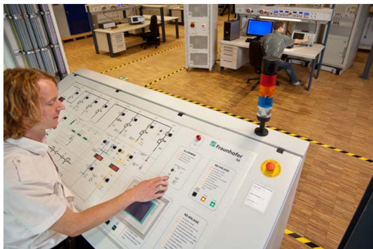
Photo 2: Control panel for the "Low-Voltage Ride-Through" test facility for testing inverters according to the new medium-voltage grid codes. ©Fraunhofer ISE
