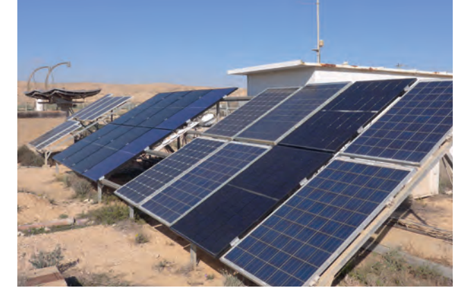
Test stand on the grounds of Ben-Gurion University of the Negev, Sede Boqer, Israel.
