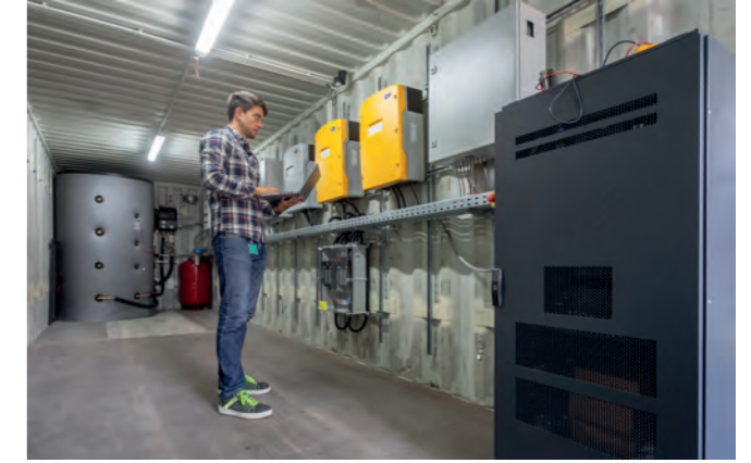
Commissioning of a cross-sectoral (electrical power, heat, cold) off-grid container. © Fraunhofer ISE/Photo: Dirk Mahler
