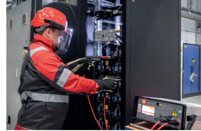
Electrical testing of high-voltage systems in our battery test laboratory. © Fraunhofer ISE/Photo: Dirk Mahler
