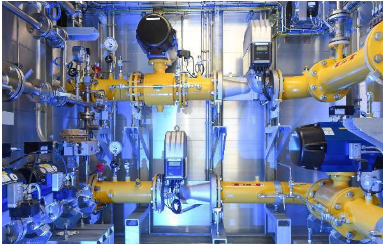
Electrolysis and H 2 Infrastructure
