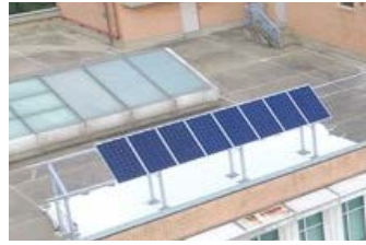
Figure 2: (System 1) Single string with 8 bifacial modules on the roof of Korea Polytechnic University
