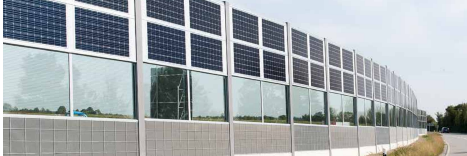
PV noise barrier in Altötting, Germany. © R. KOHLHAUER GmbH
