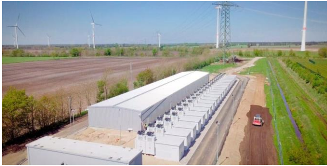
Abb. 11 Batteriespeicher Jarjelund (pv magazine, 2022)
